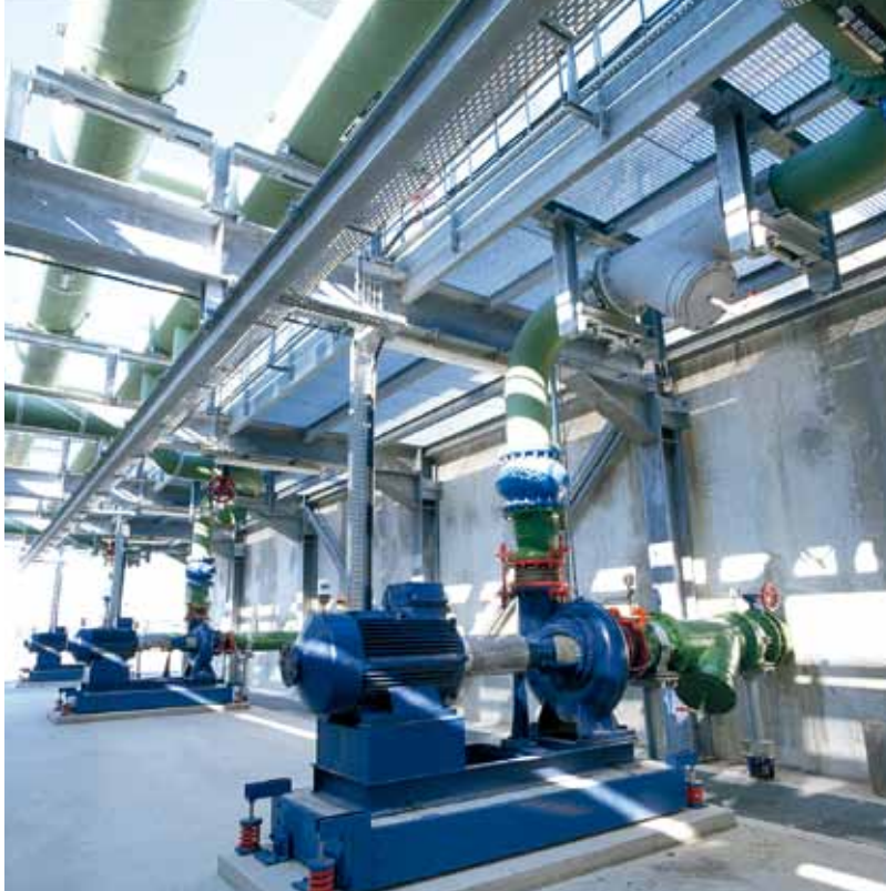
Cooling tower fan system
