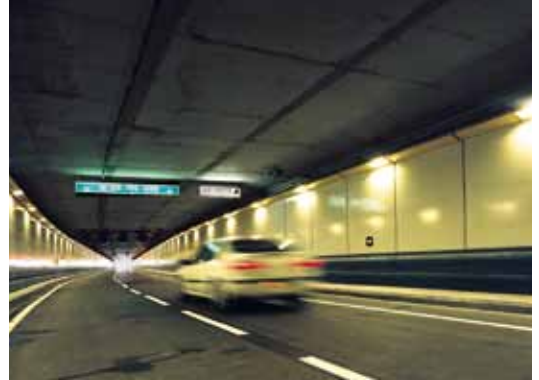
Air purification and smoke extraction system in a road tunnel
